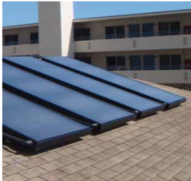
Solar thermal collector
