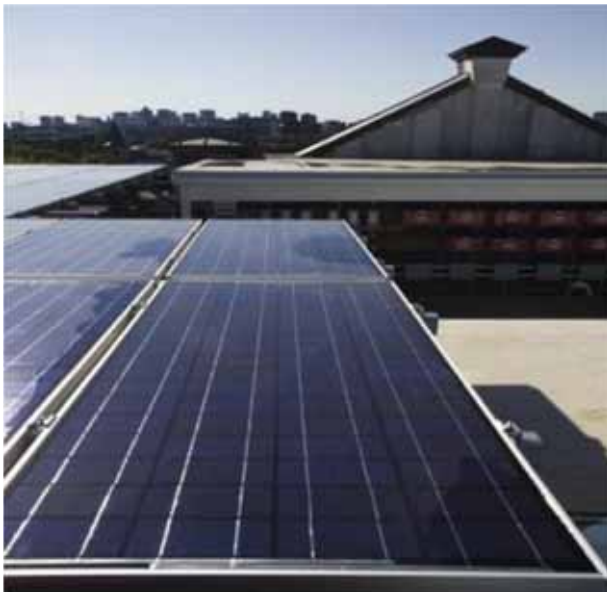
Solar photovoltaic panel
