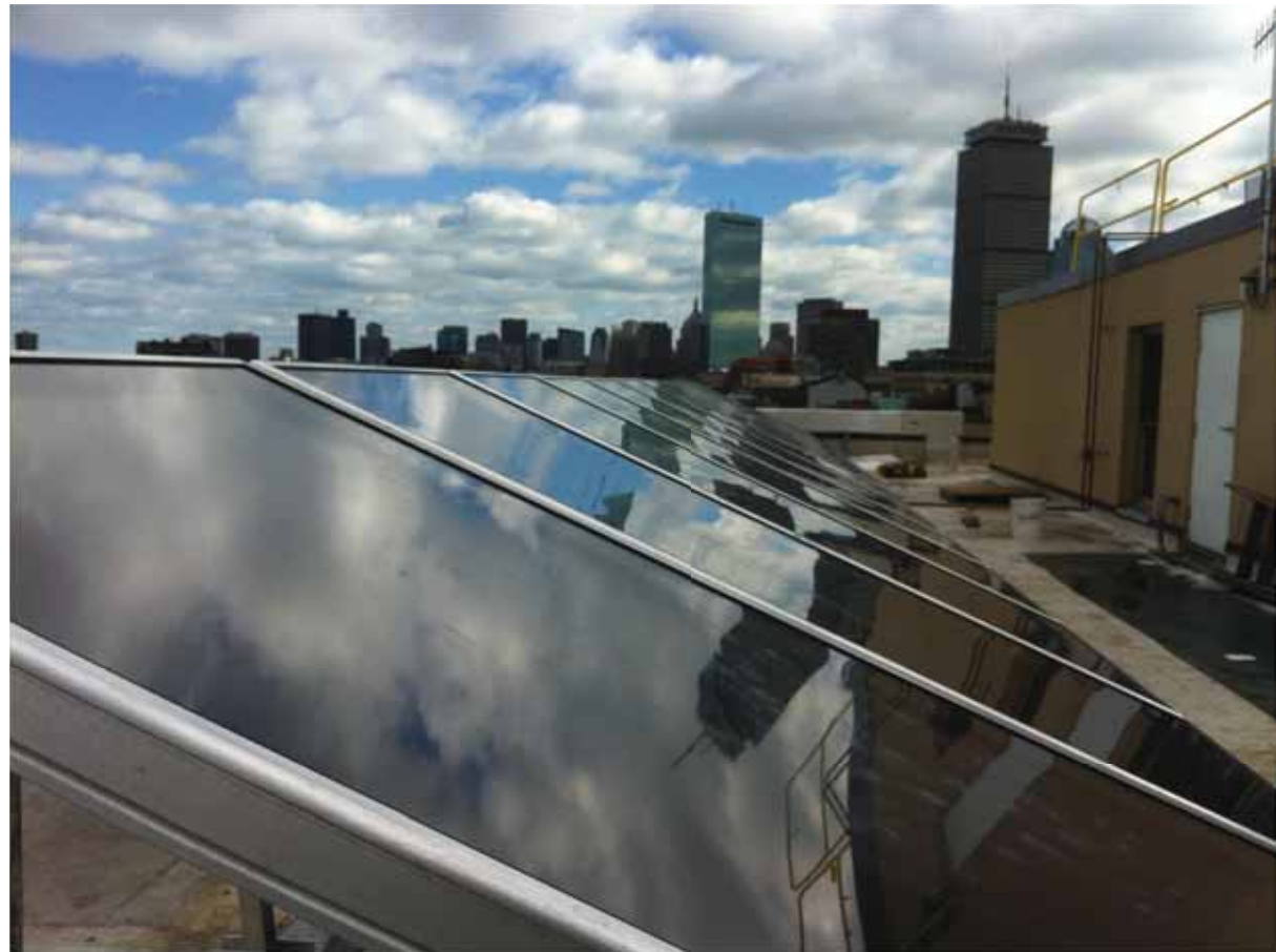
Flat-plate solar collectors
